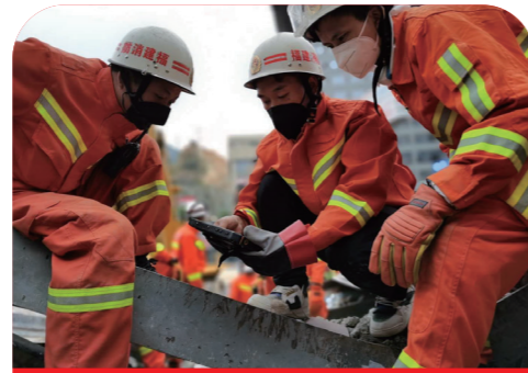
FUJIAN QUANZHOU HOTEL COLLAPSE
