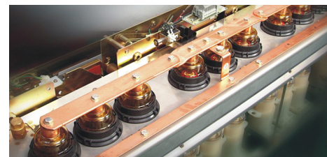
Earthing busbar system
