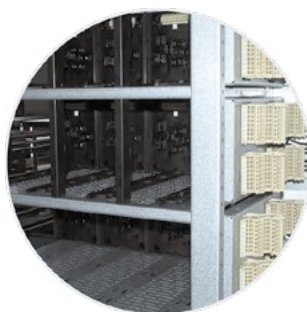
8E/4~8E/2 cabinet view
