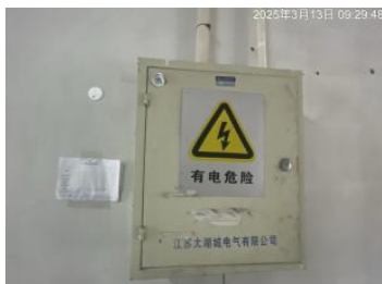
Electronic box with warning sign.JPG
