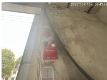
Fire alarm with backup power.JPG
