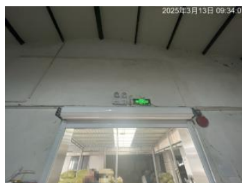
Safety exit sign, emergency light and fire alarm.JPG
