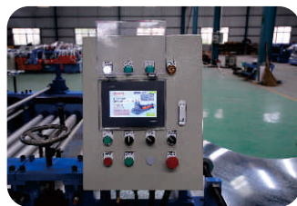
PLC 控制柜 PIC Control Cabinet
