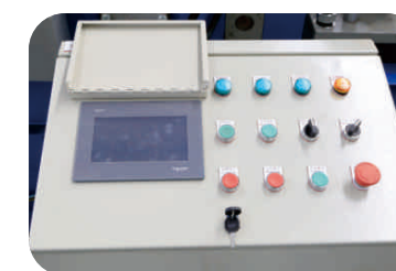
PLC 控制柜 PLC Control Cabinet
