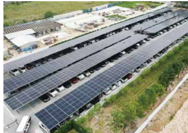
| Hospital Carport in Chon Buri, Thailand 632kW
