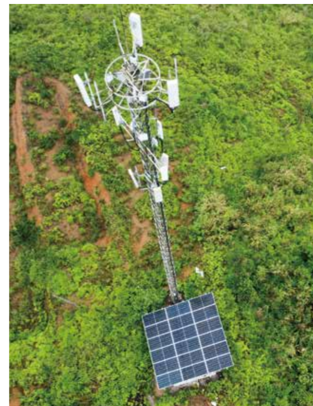
| Tieta Base Station in Jiangxi, China 12kW
