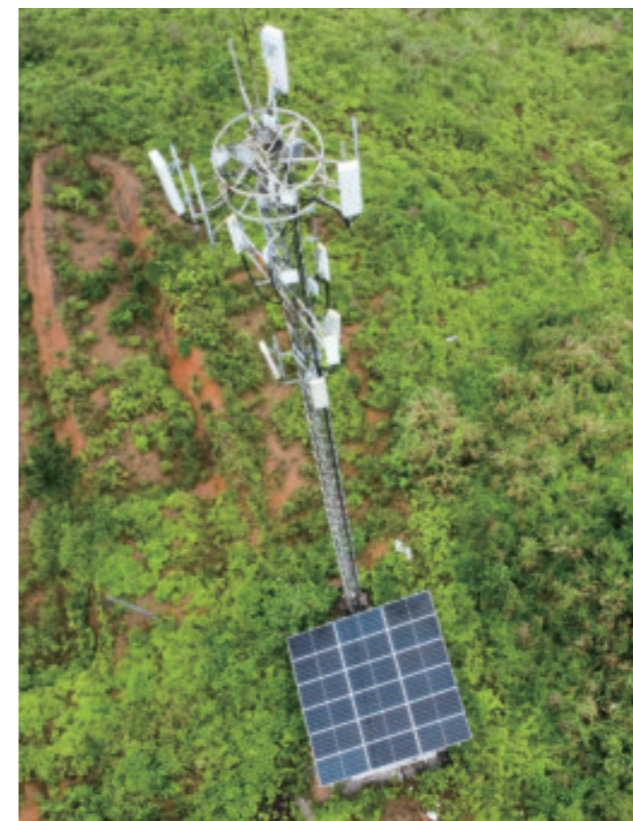
| Tieta Base Station in Jiangxi, China 12kW
