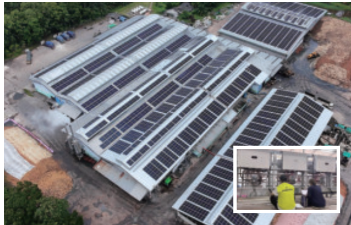
| Rubber Factory in Krabi, Thailand 2MW
