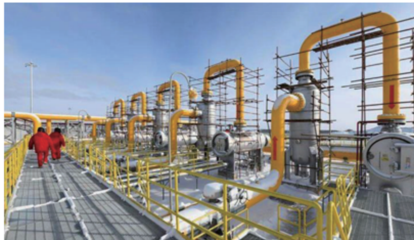
China-Russia East-Route Natural Gas Pipeline
