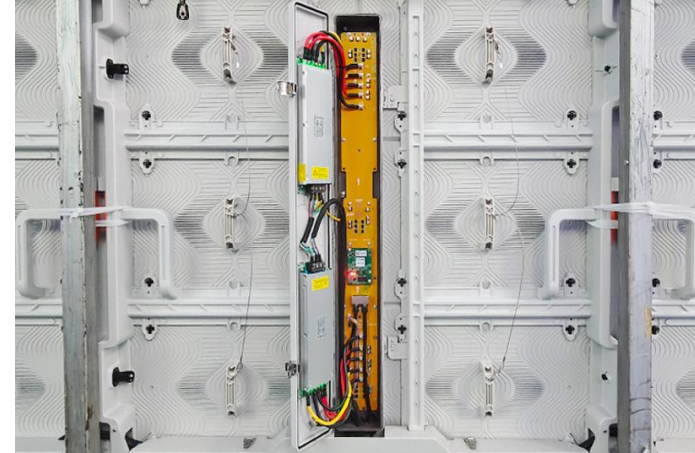
Maintenance of the power supply, receiver card, HUB board, etc.
