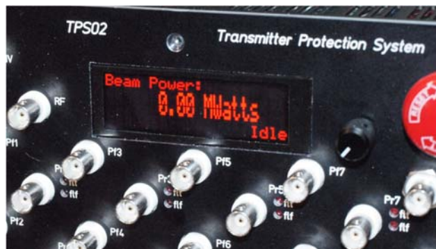
Figure 6. Top level display shows one of several parameters, and the system status in the lower right corner.
