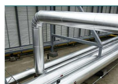
Insulated pipes 保温管道
