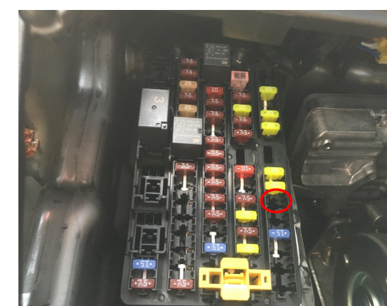
21. The fuse box is located at the driver's area and the fuse slot for power supply is indicated above.
