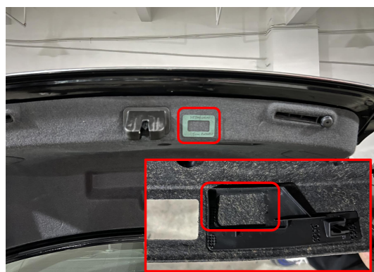
32. Stick the hole template to the indicated position, pay attention to align with the reserved empty space and open a hole for the added tailgate switch.
