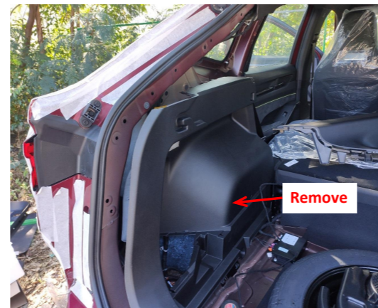
4. Remove the trunk floor mat, storage box and the indicated trim panel to allow wiring harnesses to pass
