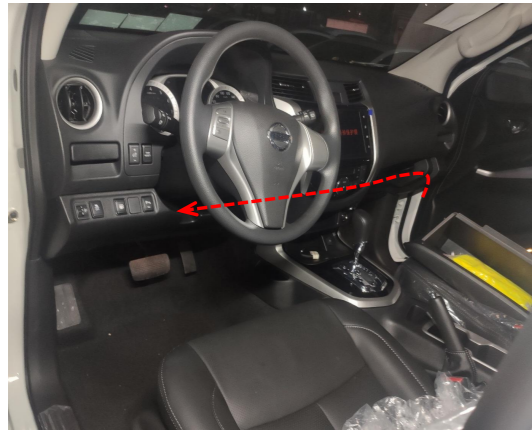
22. Route the switch wiring harness of the power harness to the driver's position.
