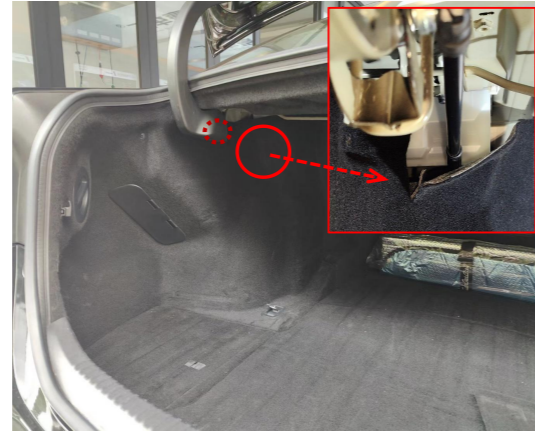
23. Reinstall all the trim panels (properly cut off the trim panels of the trunk and the hinges).
