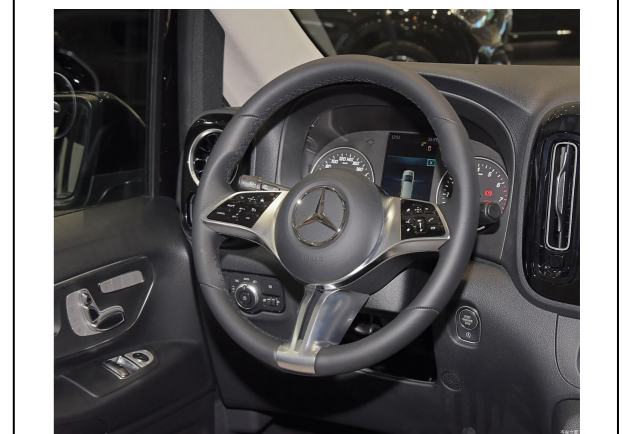
(Optional) Find an appropriate position in the driver's area, drill a \phi 21\text{mm} hole and install the added front switch.
