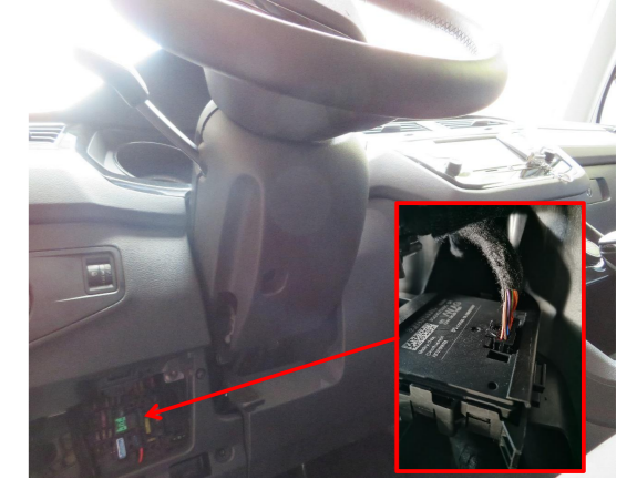
21. Find out the CAN box behind the storage box and connect to the indicated plug and its socket.
