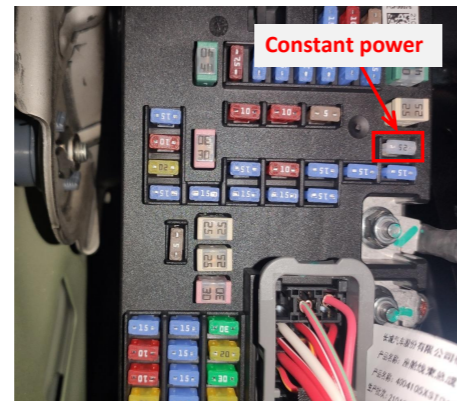
23. The fuse slot for power supply is indicated above.
