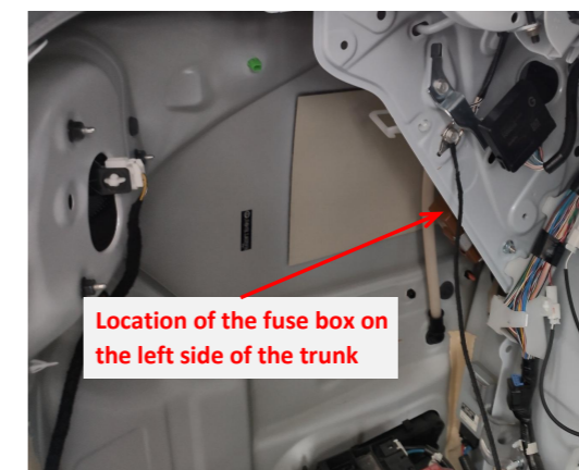
15. The fuse box located at the left side of the trunk is used for power supply.
