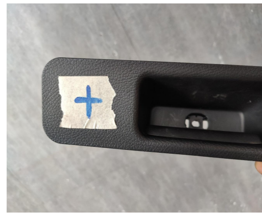
25. Stick to hole template to the indicated position of the handle and open a hole for the added tailgate switch.
