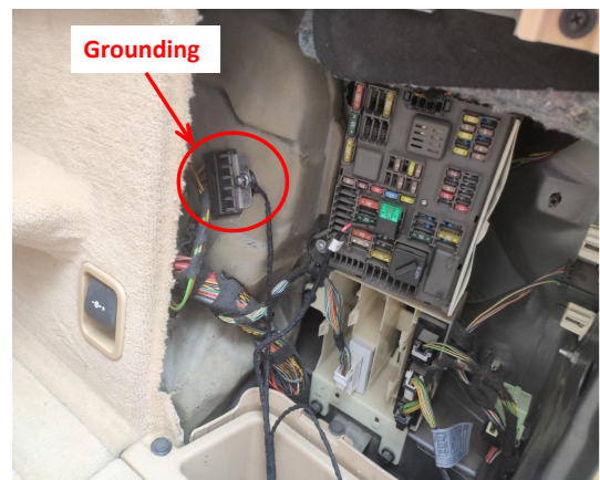
12. Ground at the right side of the trunk with the ground wire connector.
