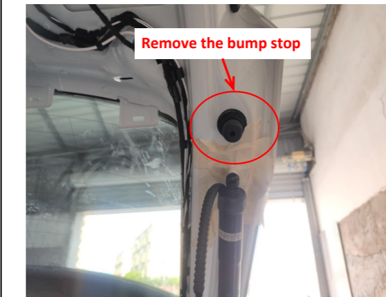
10. Remove the left and right bump stops and thread the strut wiring harnesses into the tailgate through the holes.
