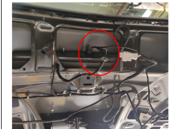
15. Connect the lock signal harness to the plugs of the original tailgate switch and the added tailgate switch.
