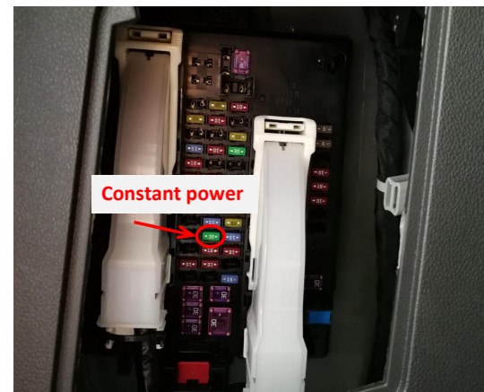
22. The fuse slot for power supply is indicated above.
