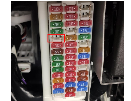
23. The fuse box is located beside the pedals and the fuse slot for power connection is indicated above.
