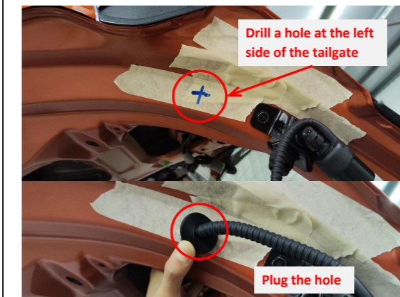
8. Drill a hole at the right side of the tailgate and plug the hole securely.
