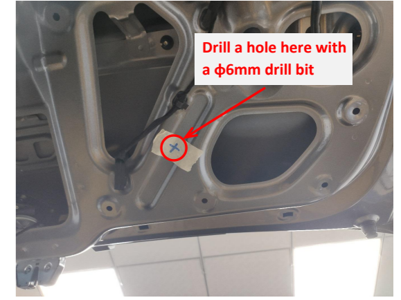
21. Drill a hole at the indicated position with a φ6mm drill bit, fix the ECU to the hole and secure it with a nut.
