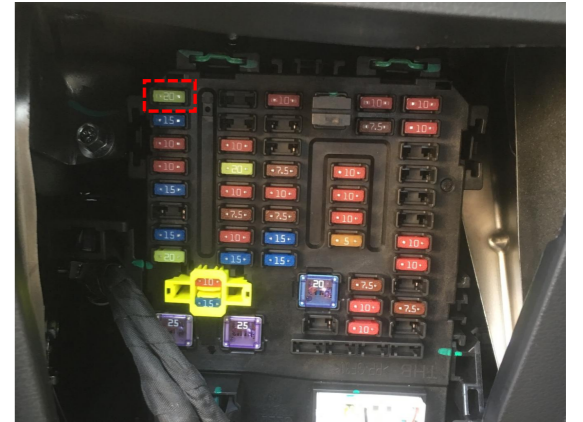
21. The fuse slot location of constant power (first in the first row).
