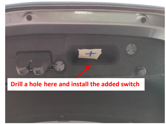
31. Drill a hole at the indicated position with a φ20mm drill bit for the installation of the added switch.
