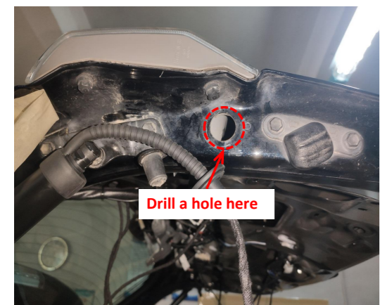
12. Use a φ21mm drill bit to drill a hole at the indicated position of tailgate. Both sides are the same.
