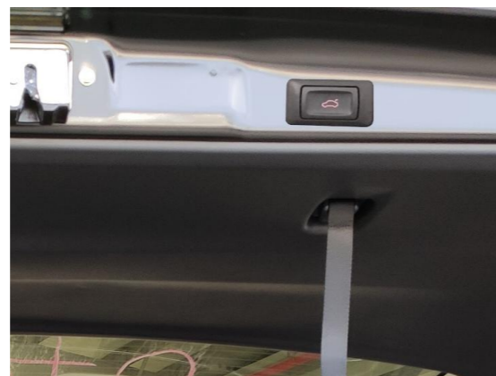
33. Reinstall all the trim panels and fit the added tailgate switch in.
