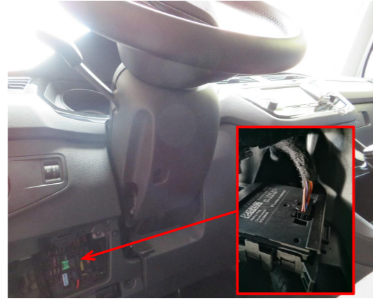
18. Connect the power harness to the indicated signal plug behind the fuse box.
