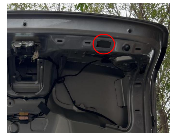
26. Open a hole at the indicated position with a φ21mm drill bit for the added tailgate switch.
