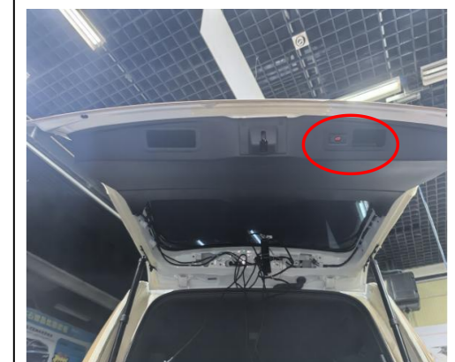
38. Remove the original tailgate handle, install the added tailgate switch and reinstall all the trim panels.
