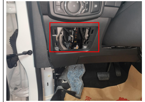
20. Find out the fuse box in the driver's area for power supply.
