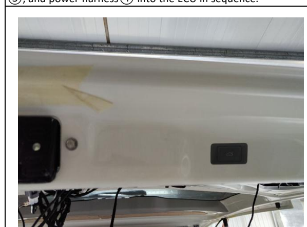
32. Reinstall all the trim panels and fit the added tailgate switch in.
