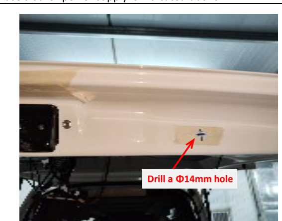
30. Drill a hole at the indicated position with a Φ14mm drill bit.
