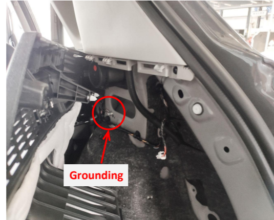
23. Ground at the indicated position on the right side of the trunk.
