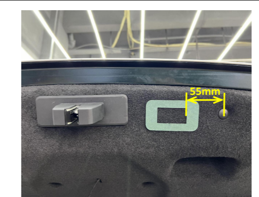
30. The location of added tailgate switch is as shown above. Stick the hole template here and open a hole. The hole should be align with the hole of sheet metal.
