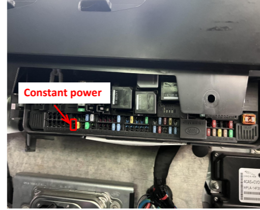
19. The fuse box is located at the right side of the trunk.
