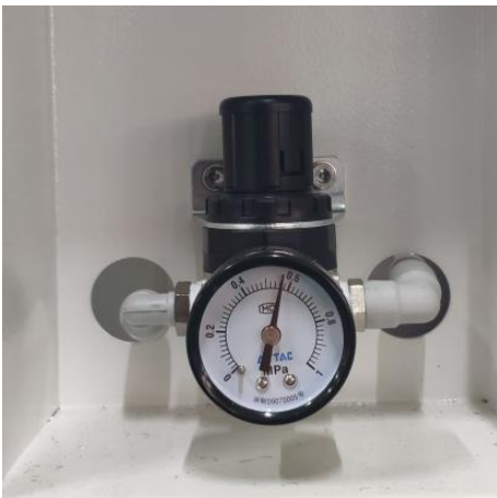
Fig E- Feeder air pressure value pressure 0.5MP
