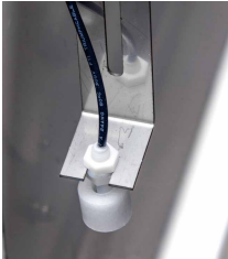
Water level sensor
