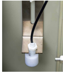
Water level sensor
