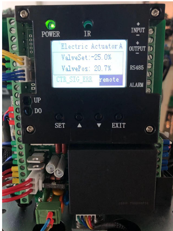
Figure 4 electrical control module
