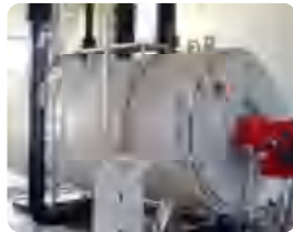
• Steam Boiler 蒸汽锅炉
