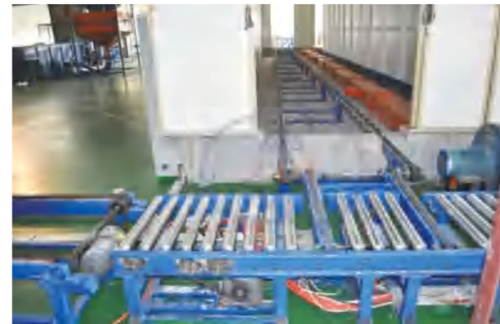
EPS/EPP drying room
