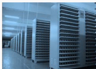
Battery Test Equipment
