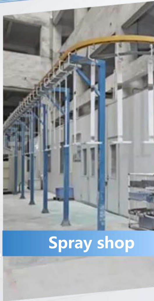
Automatic infiltration line
