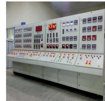
Industrial Control Equipment
