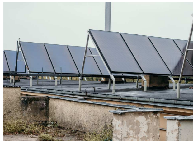
May 2021 – Slovenia – 200 pieces – comprehensive power generation increased by 10.8%
