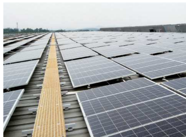
PV System Project Fukuoka, Japan | Year: 2021
