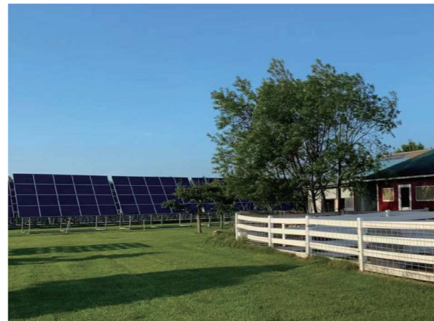
PV System Project Hokkaido, Japan | Year: 2022
