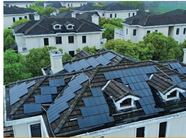
PV System Project Suzhou, China | Year: 2020
