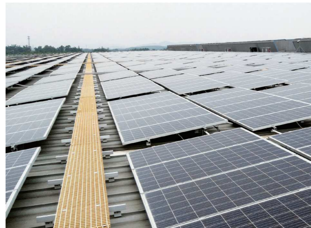
PV System Project Fukuoka, Japan | Year: 2021
